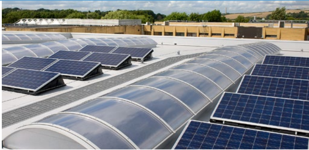
Solar photovoltaic roof panels and sun pipes installed at the Shoreham Technical Centre generate 4752 kWh of extra electricity and save 2.6 tonnes of carbon per annum
