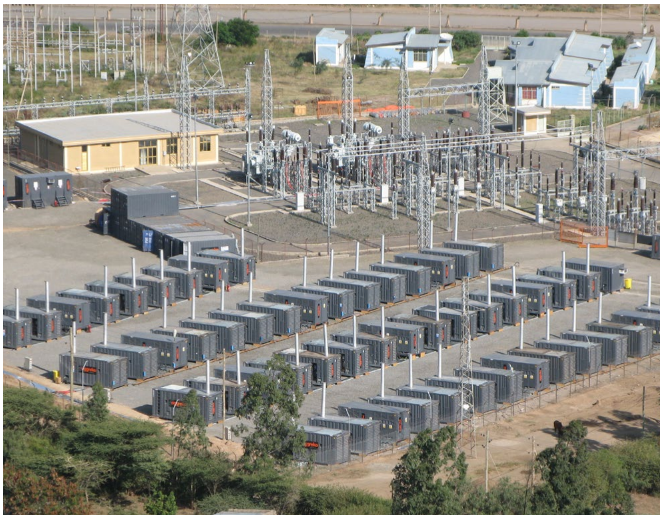
Aggreko's strategy has been to expand its global presence by making temporary power cost-competitive with permanent generating plant. Pictured above is a 30 MW Aggreko power project in Ethiopia
